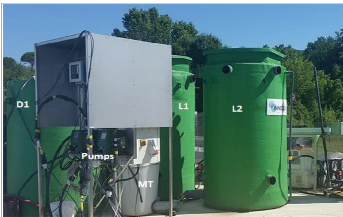
Figure 5.12. INNOQUA integrated system at the UDG pilot-site (Quart WWT, Girona, Spain). The system consisted of two 5 PE lumbrifilters (L1 and L2), a mixing tank (MT) and a 10 PE Daphniafilter (D1).
