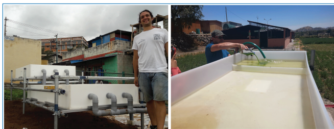
Figure 6.9. Pilot-scale BSP modules of the INNOQUA system installed in India (left) and Peru during inoculation (right).
